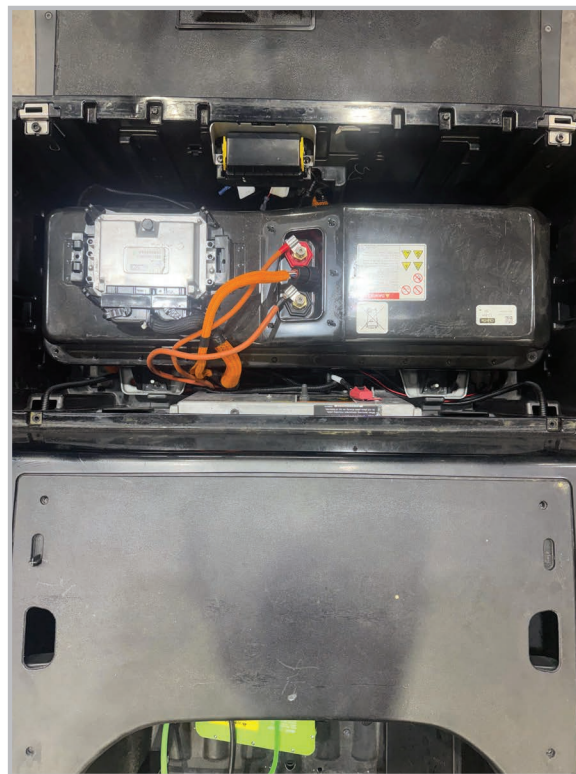
LG factory battery installed under the seat – VCM, HV cables, and terminals
